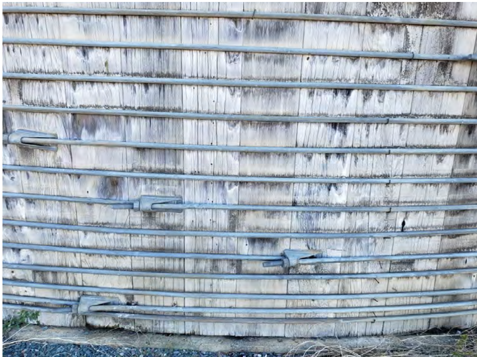
View of redwood tank wall, showing overall integrity, spacing of metal bands and fasteners, and interface with concrete platform underneath, taken 11/10/22, Photo #1135810, from Photolog BS-01.
