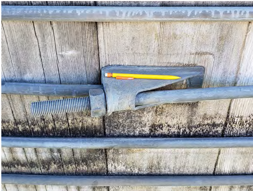
Close-up of metal fasteners which hold redwood tank's metal bands, facing east, taken 11/10/22, Photo #133756, from Photolog BS-01.
