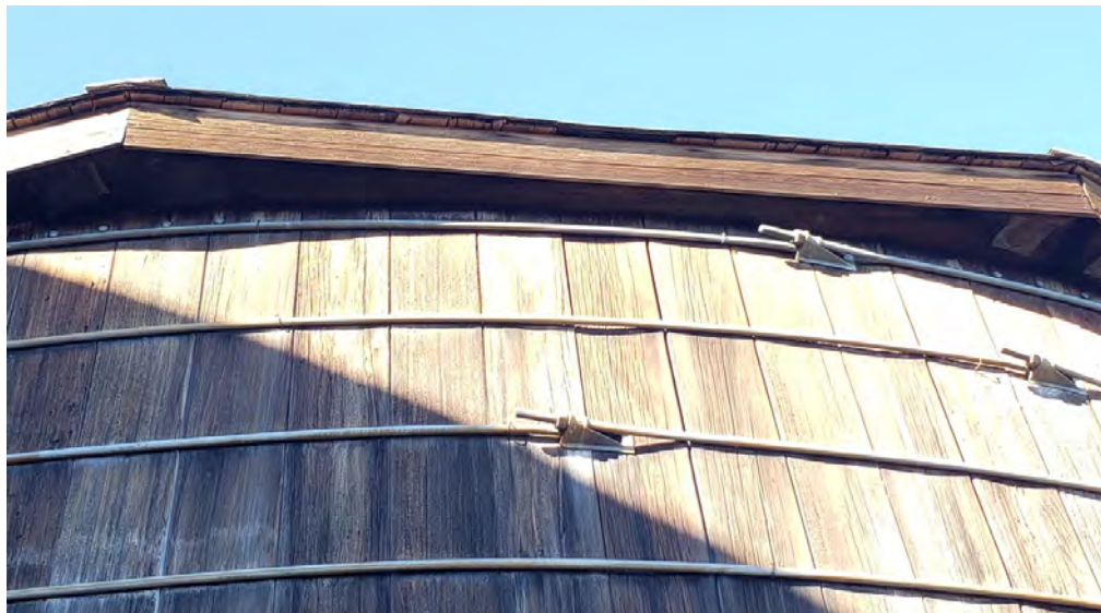
Close up #1 of redwood tank roof construction, showing wooden planks radiating outward from center of roof, and wooden planks which form the perimeter of the structure, taken 11/10/22, Photo #135202, from Photolog BS-01.
