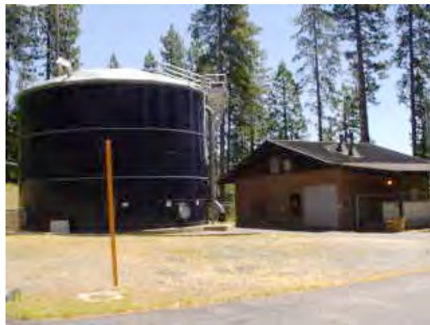
Meadowmont Tank and Pumping Station
