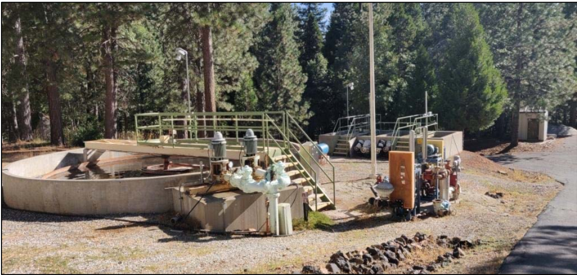
Secondary Clarifier, Filter Feed Pump Pump Station, RAS/WAS Pump Station Aerobic Digesters in Distance
