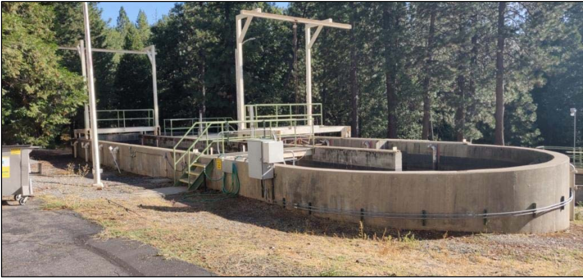
Arnold WWTF Oxidation Ditch
