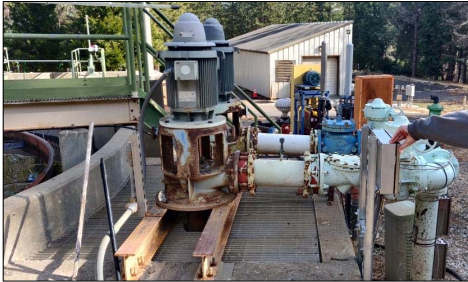
Filter Feed Pump Station – Pumps No. 1 and 2
