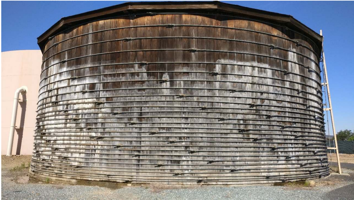
Figure 6. Condition of B Tank #1
