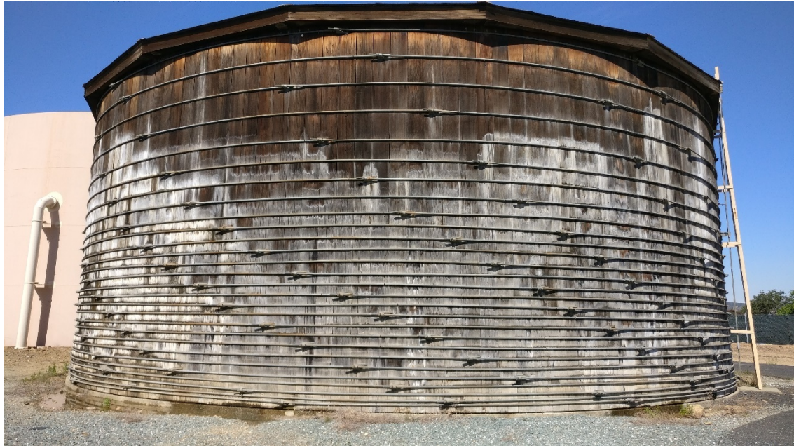
Figure 6. Condition of B Tank #1
