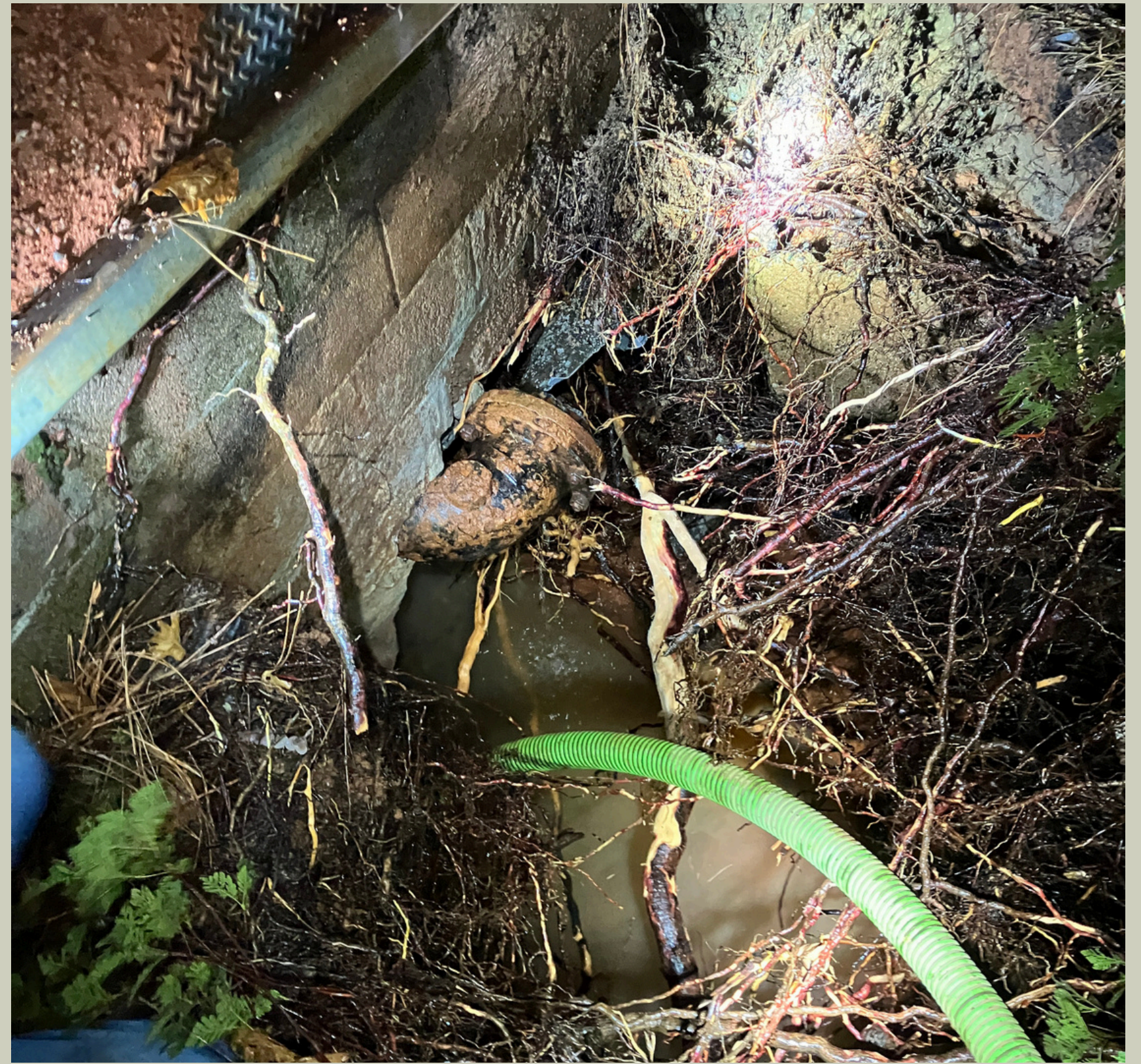
Leak at PRV 30 on Thunderbolt - Ebbetts Pass
