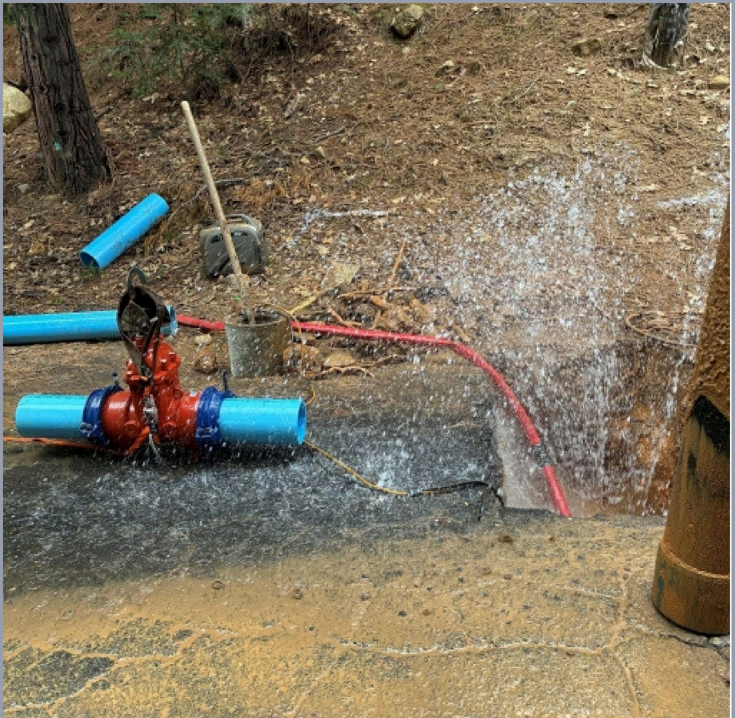
Fixed a leak on the Reclaimed Water line - Vallecito Installing an inline Valve in Big Trees Village
