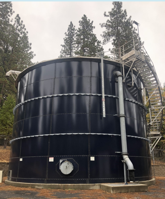
Recently constructed CCWD water tank located in the Meadowmont subdivision of Arnold.
